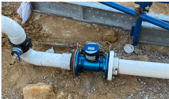
Electromagnetic flow meter and sample point
