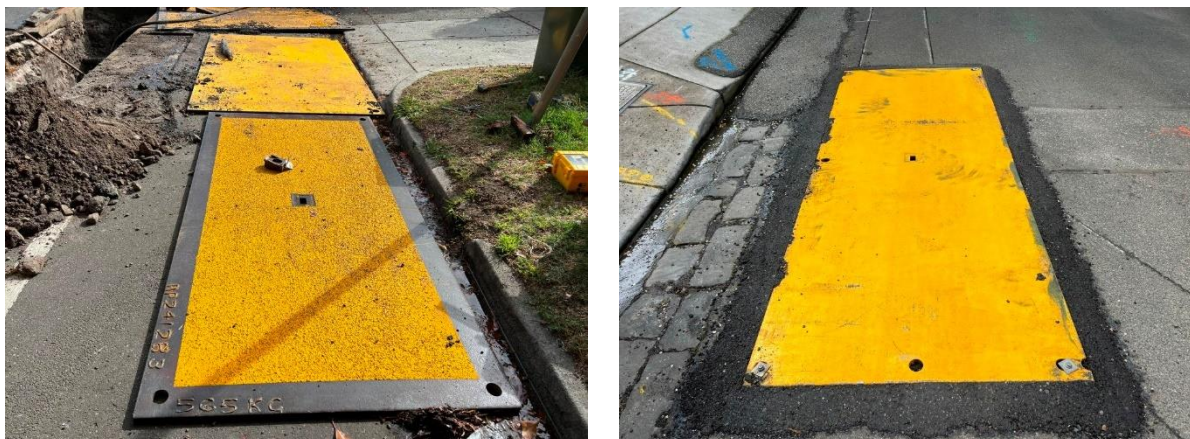
Figure 10: Compliant road plates over open excavations on South East Water projects
