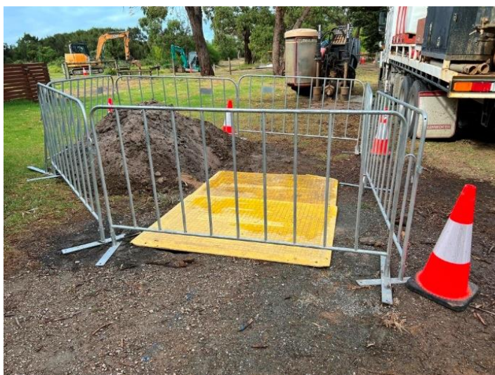
Figure 11: Compliant plastic cover over an open excavation on a South East Water project
